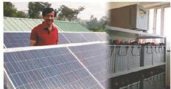
Rotary Installation, Bangalore - Solar PV Offgrid 9000Wh System
